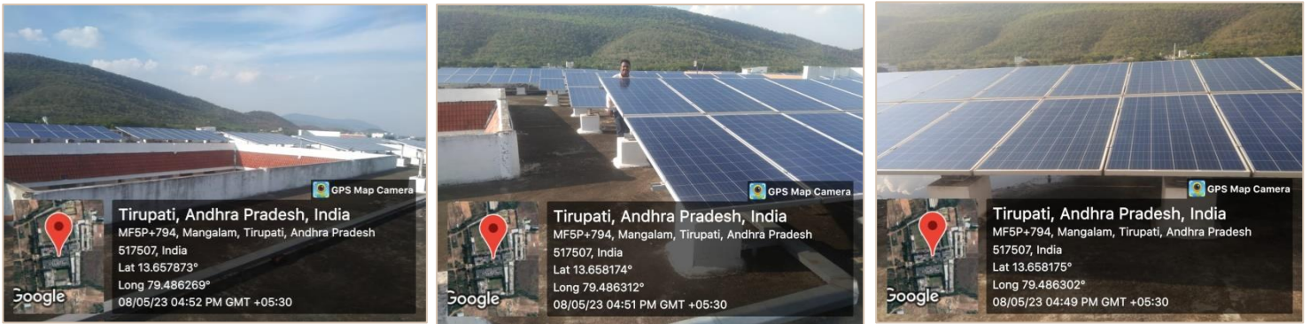
Investigative parameters – Energy Management – Solar panels in the premises
